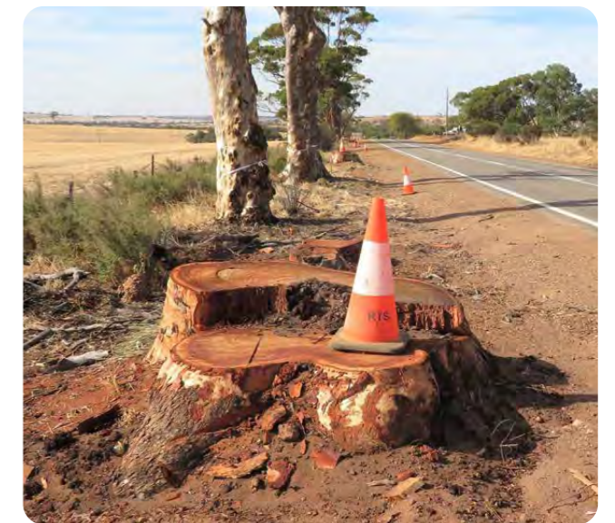
Large mature tree cut down by Main Roads. Image by Brett Loney.
